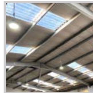
GRP Roofing Lights
